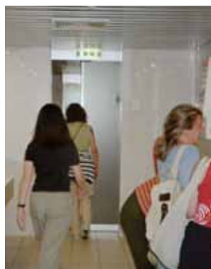
Automatic sliding door, sanitary area, ZRH
