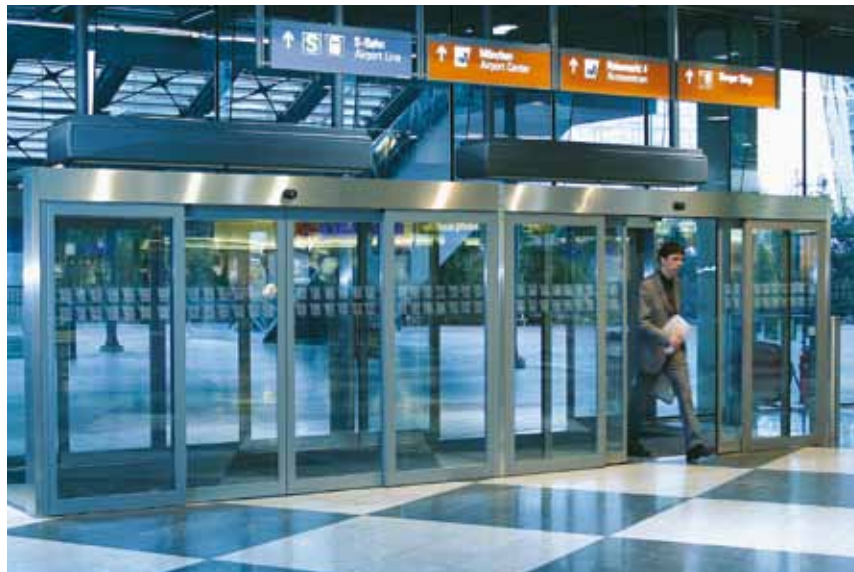
Smoke-protection doors, entrance area, MUC
