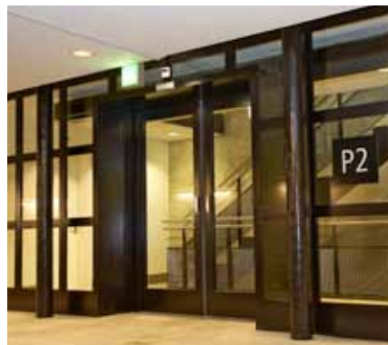
Automatic smoke-protection door, multi-storey car park
